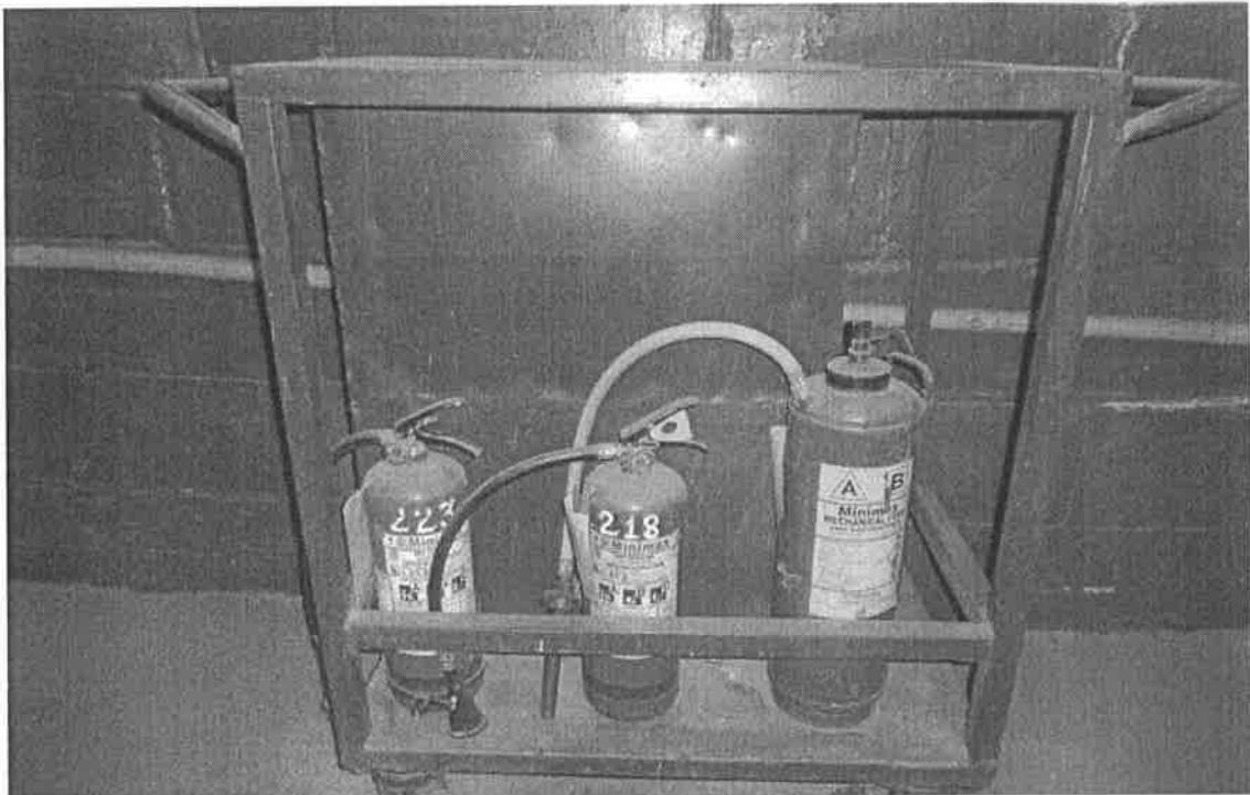
PORTABLE EXTINGUISHERS ON TROLLEY
