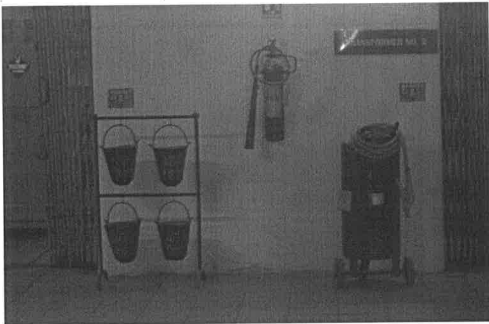
SAND BUCKET WITH FIRE EXTINGUISHER
