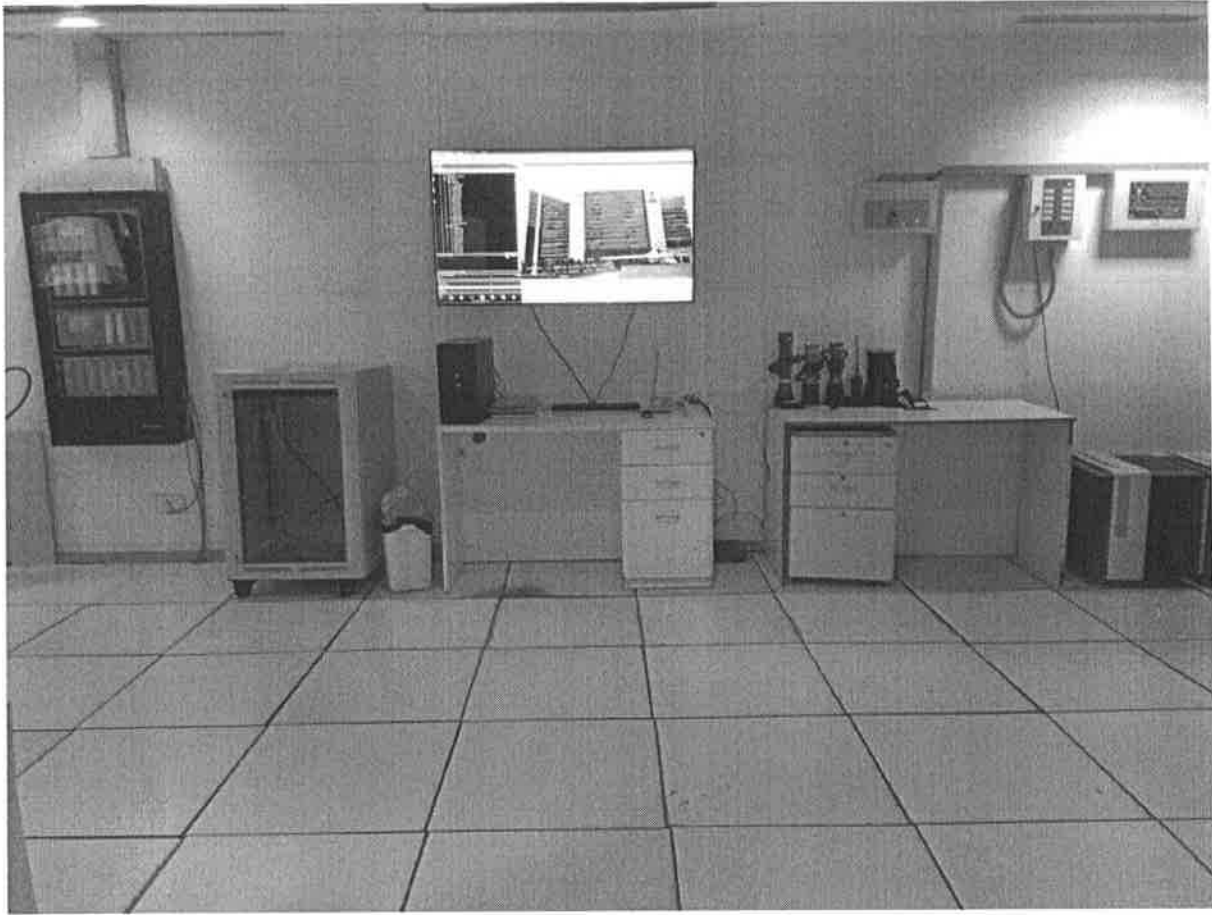
FIRE CONTROL ROOM
