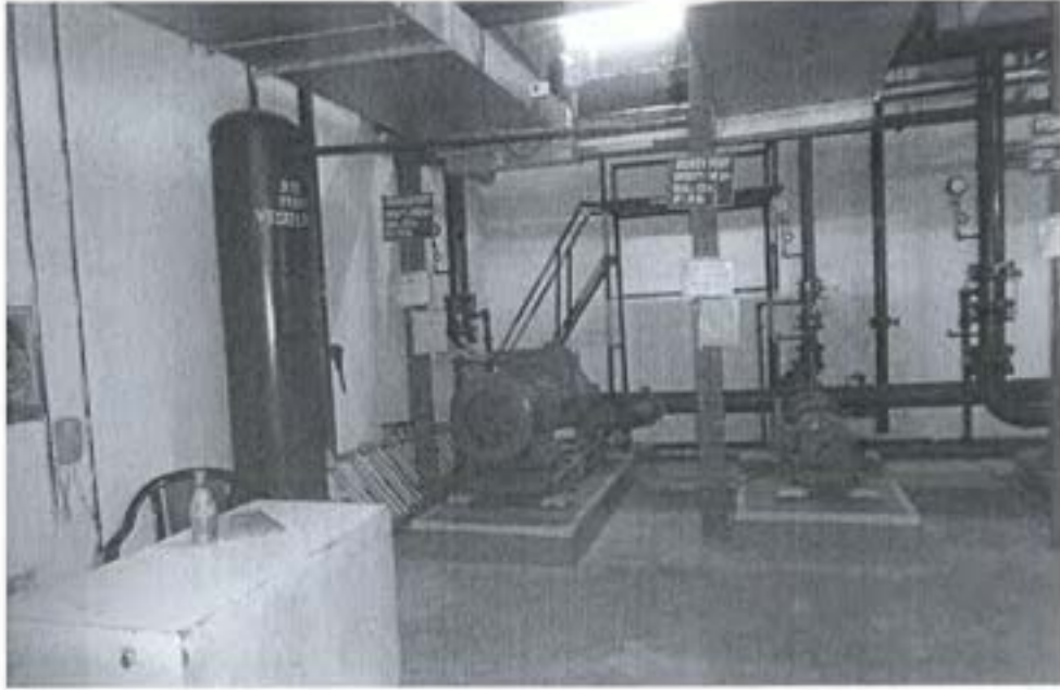
FIRE PUMP ROOM
