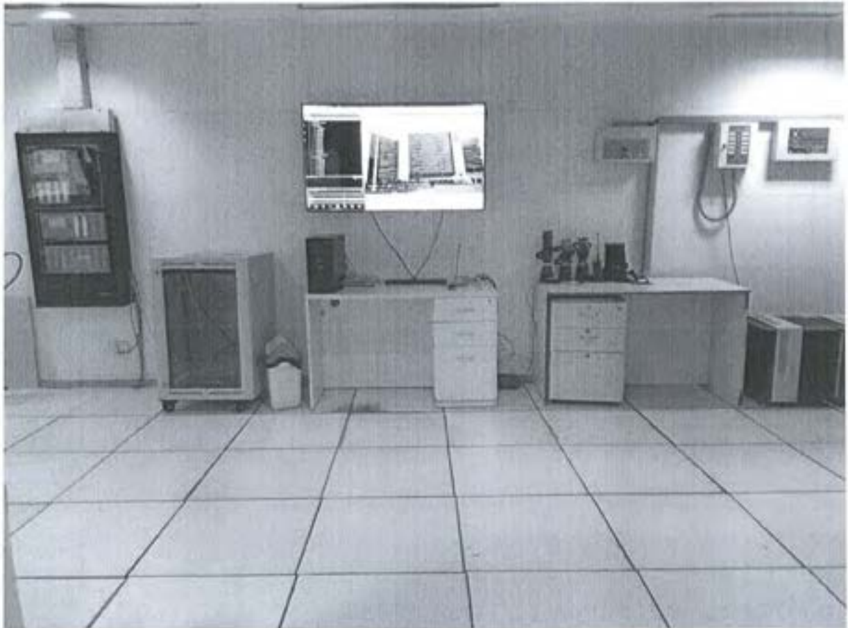
FIRE CONTROL ROOM
