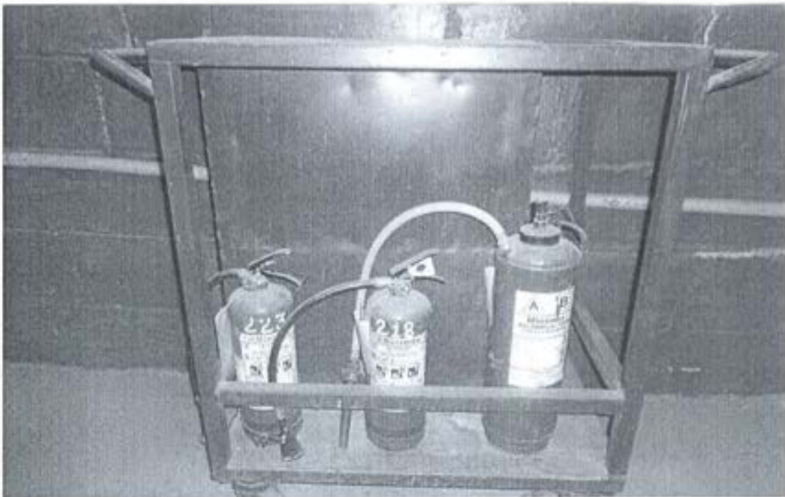
PORTABLE EXTINGUISHERS ON TROLLEY
