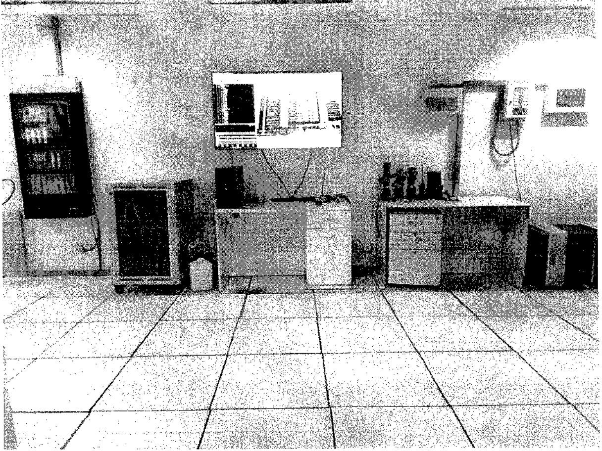
FIRE CONTROL ROOM
