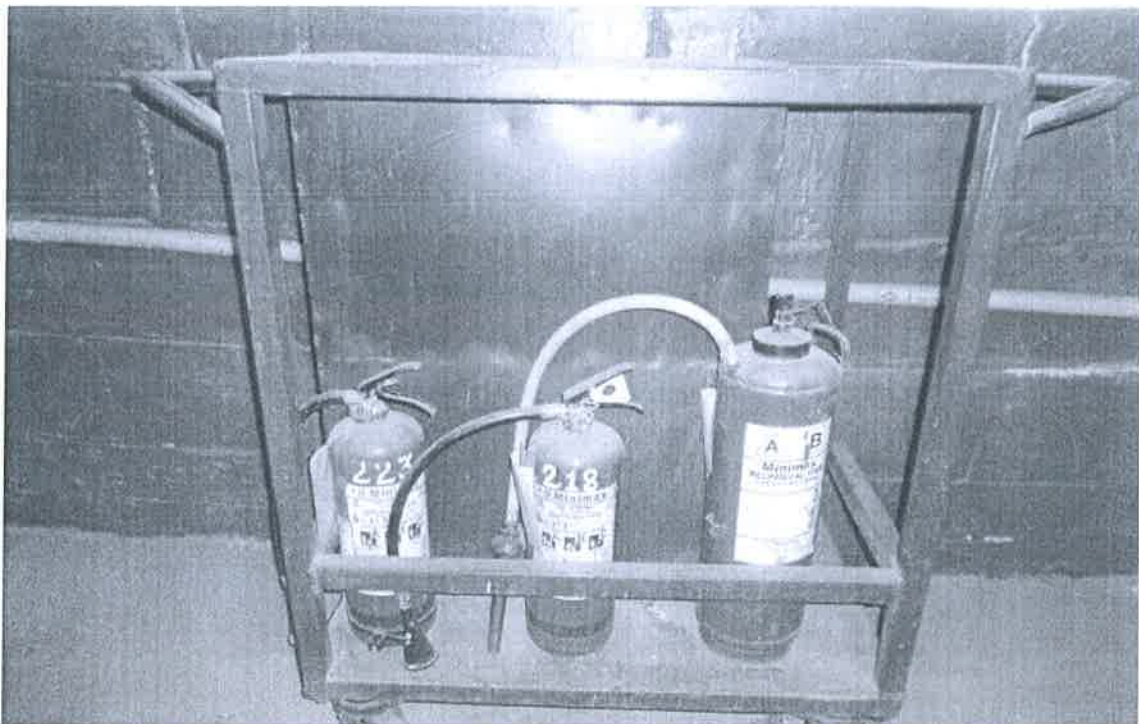
PORTABLE EXTINGUISHERS ON TROLLEY
