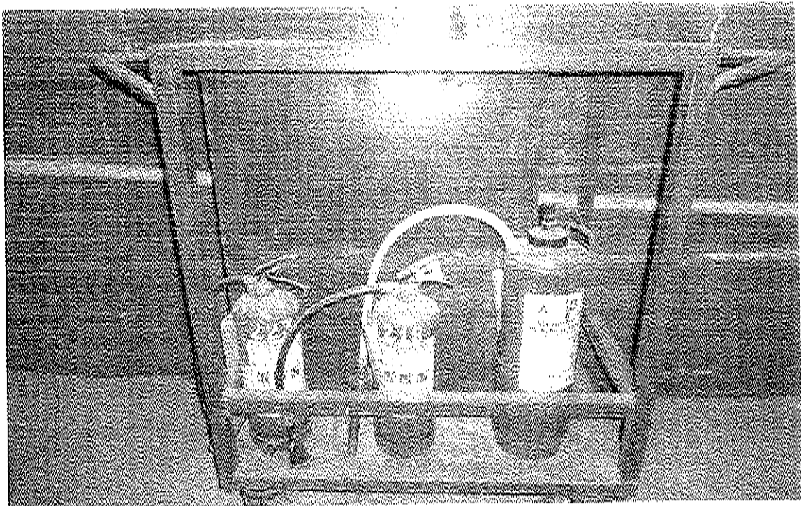
PORTABLE EXTINGUISHERS ON TROLLEY
